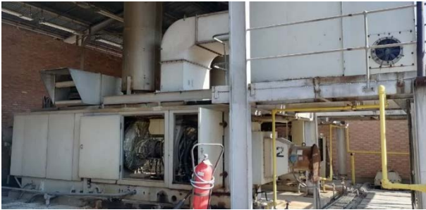
Fig. 5. Turbine generator part of the hybrid power plant is set to be installed [8].
